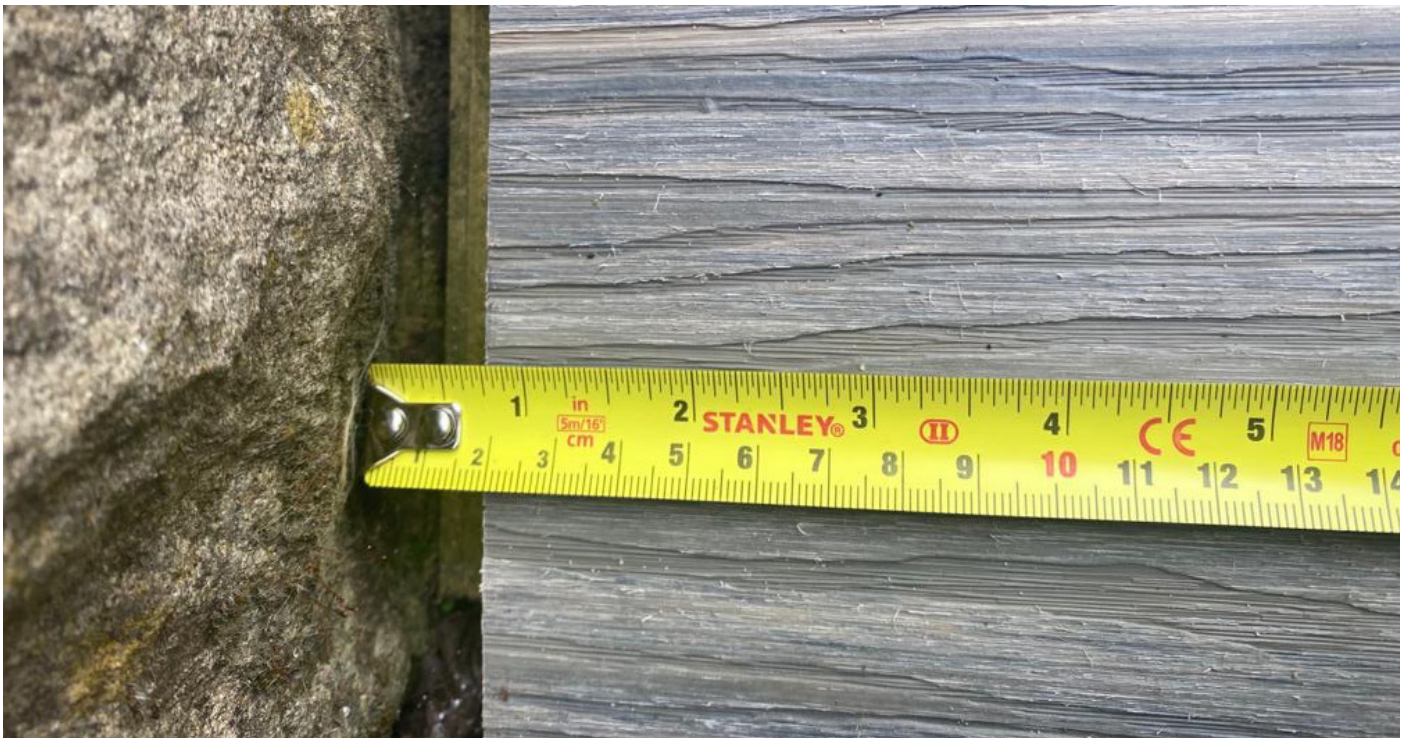
Expansion Gaps at Wall
